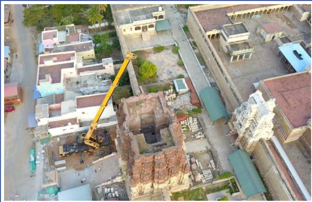
This crane from Germany can handle 300 tonnes at ground level & 30 tonnes at 150' height arrived at the temple site on Tuesday 25 December 2018
