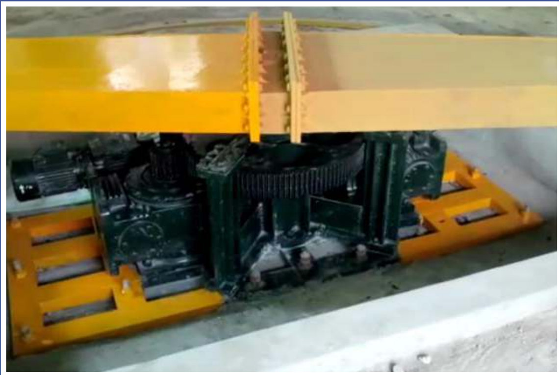
Two sets of gear boxes powered by two horse power motors each
